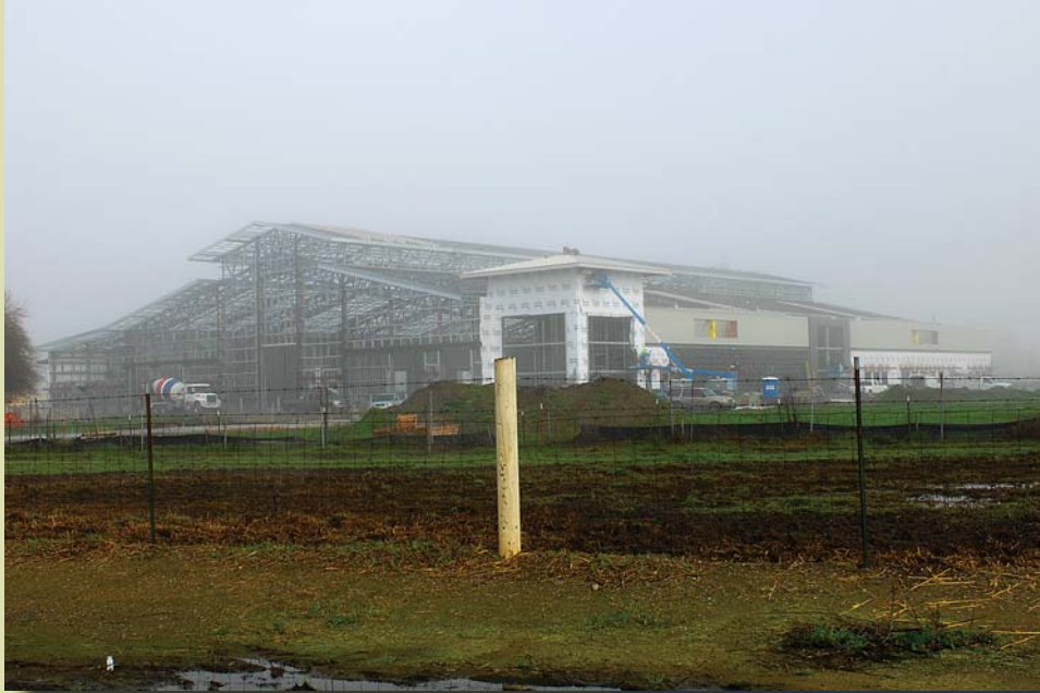
Construction on the impressive Agriculture Pavilion has been delayed due to issues with the steel fabricator. The project is now expected to be finished in August 2011.
