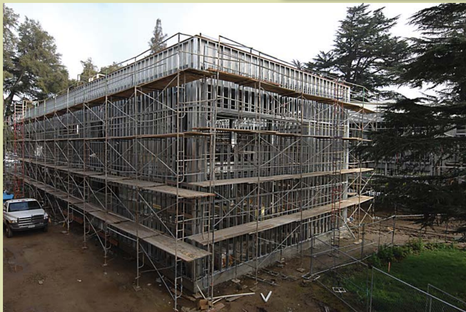
Construction of the Student Services Building continues on schedule with completion expected in October 2011.
